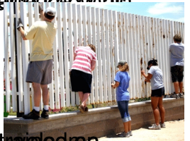
Painting the exterior of a building for a family in a Metroplex area. Photo by: [Name]
